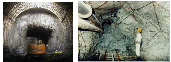
Figure 3: High rock stresses in a) weak rock results in great deformations (figure left). b) hard rock results in spalling and/or rockburst (figure right).
